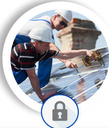
Installation Workmanship Errors
